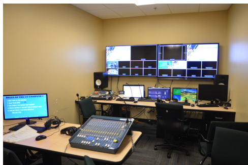
Figure 7 MUTV control room
