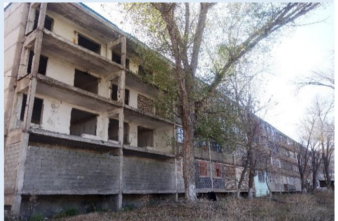
Figure 2: Damaged housing in Jaňatas
