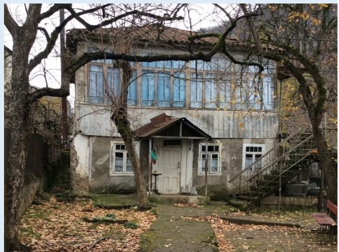
Figure 2: House in need of renovation
