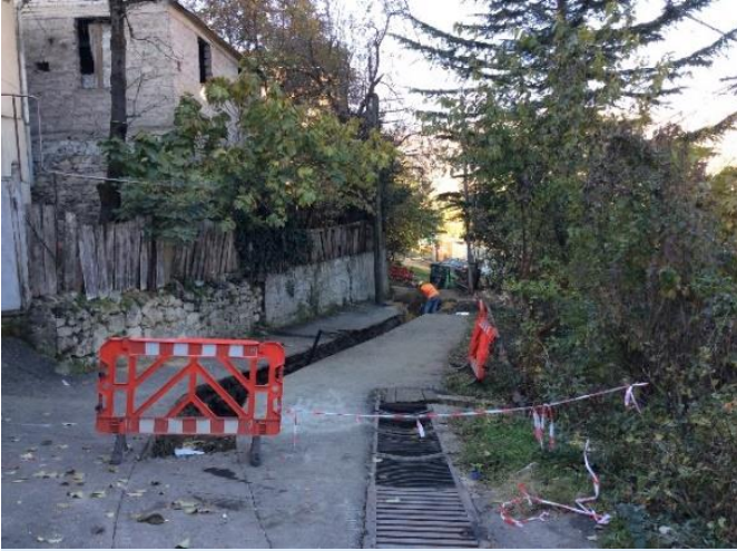
Figure 5: Deterioration of infrastructure
