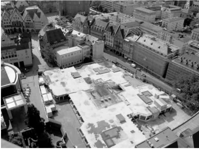
Figure 3: Cleared to build a “historic” town center. Demolition of the “Technisches Rathaus” (Photo: Sarah Bonnert, 2011)
