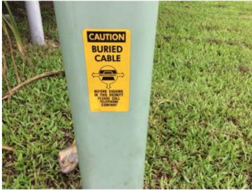
Figure 1. “Caution: buried cable. Before digging in this vicinity please call telephone company”
