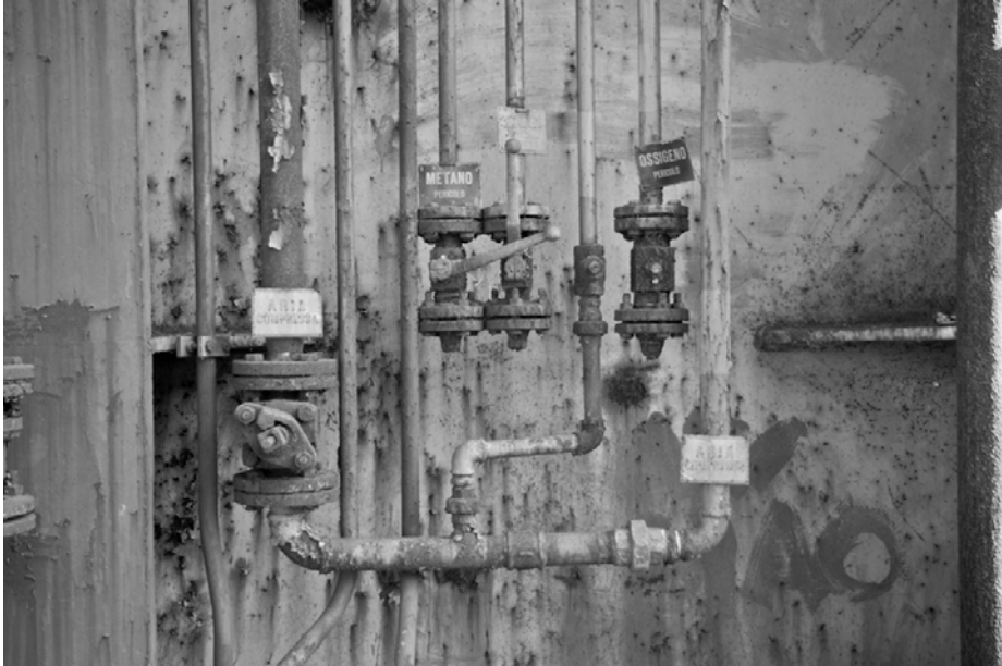
Figure 7: Compressed air and methane gas system (Photo: U. Gillio 2015)
