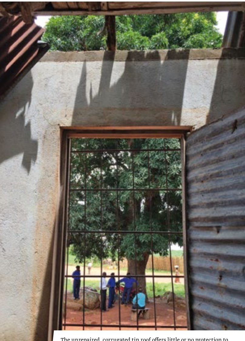
The unrepaired, corrugated tin roof offers little or no protection to the weapons or ammunition against either theft or the elements.
