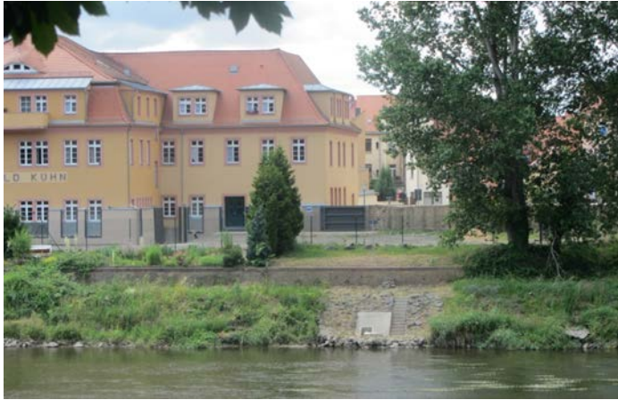
Figure 3 New floodwall, part of Project 2, with passageways for accessing the river and allowing a view (2017, authors) short notice in case of imminent floods (hochwasserschutz-grimma.de, 2017).
